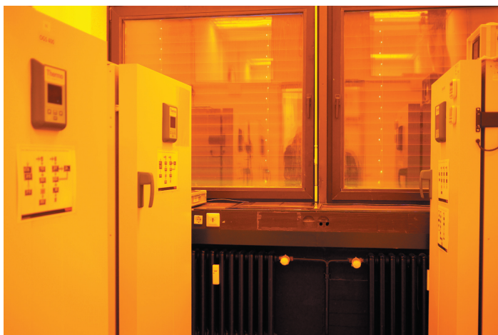
View of the heating cabinets
